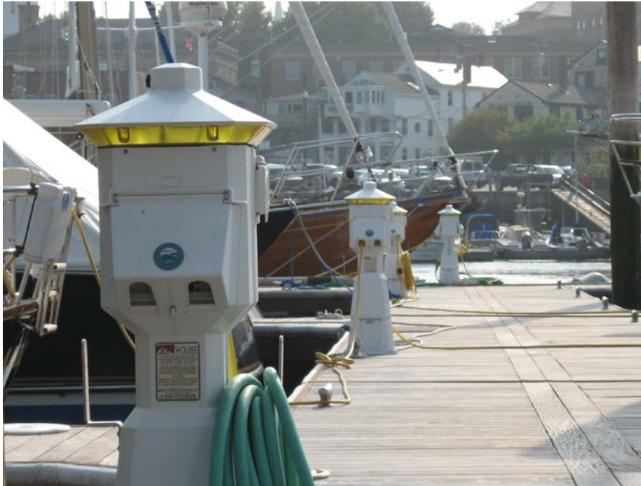
Electric power pedestals at a marina
